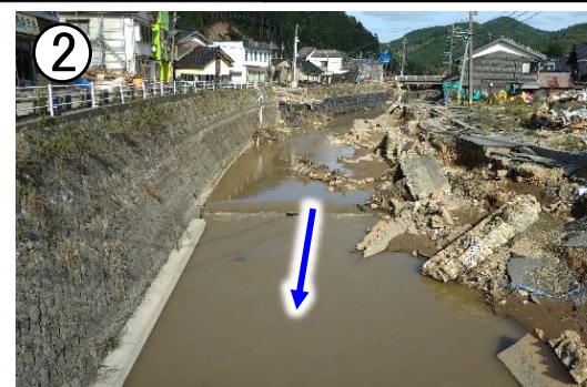
護岸の被災状況(鈴屋川)
