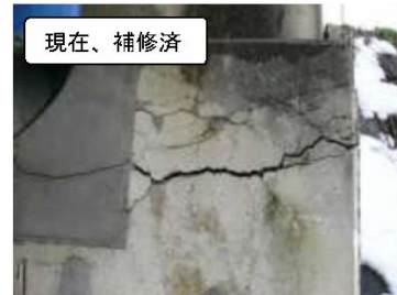
ASR劣化橋梁
